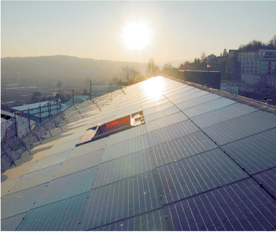
Anlage Application Application Waidspital, Zürich (CH)
