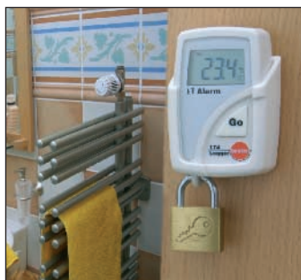
Monitoring temperature control in a radiator thermostat
