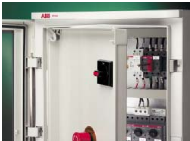
Example of the configuration of a switchboard for an automation application: some ABB control and protection devices are installed on the plate. The inner door is fitted with light-signaling devices.
