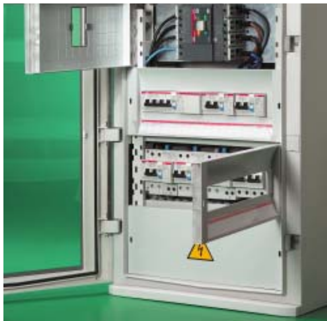
The blank and drilled panels are hinged onto both sides; the description of the installed components can be kept in the special compartment protected by a transparent, hinged flange.
